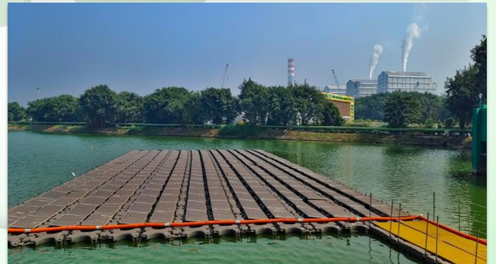
Floating Solar Panel on Reserve pond
