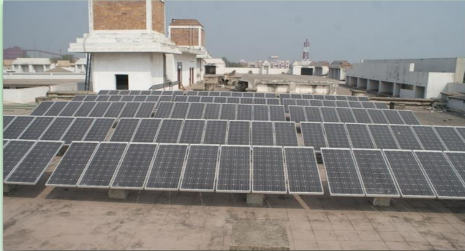
Solar Panels on Administrative Building
