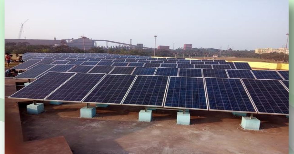
Solar Panels on Community Centre
